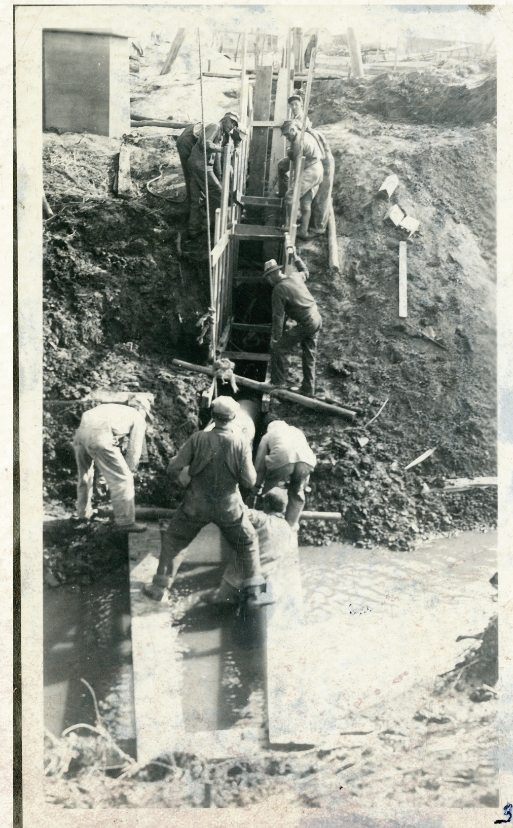
Seven men install 18-inch intake pipe in an irrigation canal at the Union Fruit Farm Pumping Plant. Date unknown.
